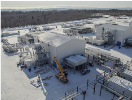
The Wilde Lake Compressor Station, located in Groundbirch, B.C., achieved mechanical completion and is ready to receive gas for the first time.
