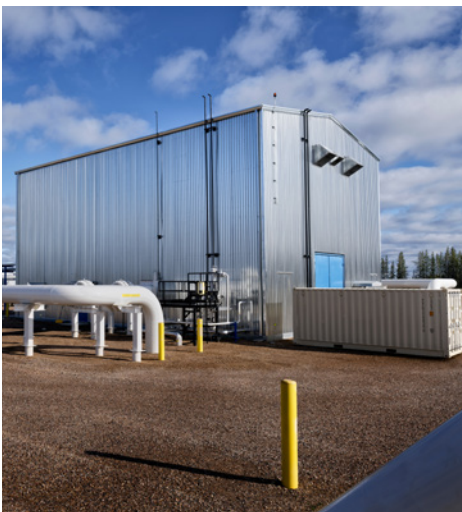
Example of a compressor station
