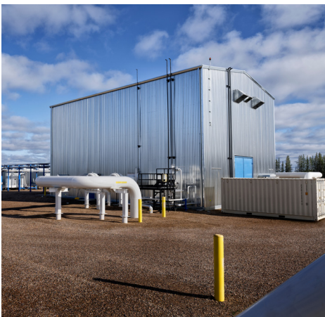
Example of a compressor station
