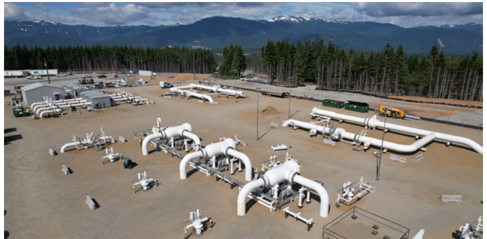
Aerial photo of the Kitimat Meter Station
