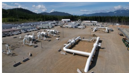
The Kitimat Meter Station, where natural gas would be inspected, measured and then delivered to the LNG Canada facility.
