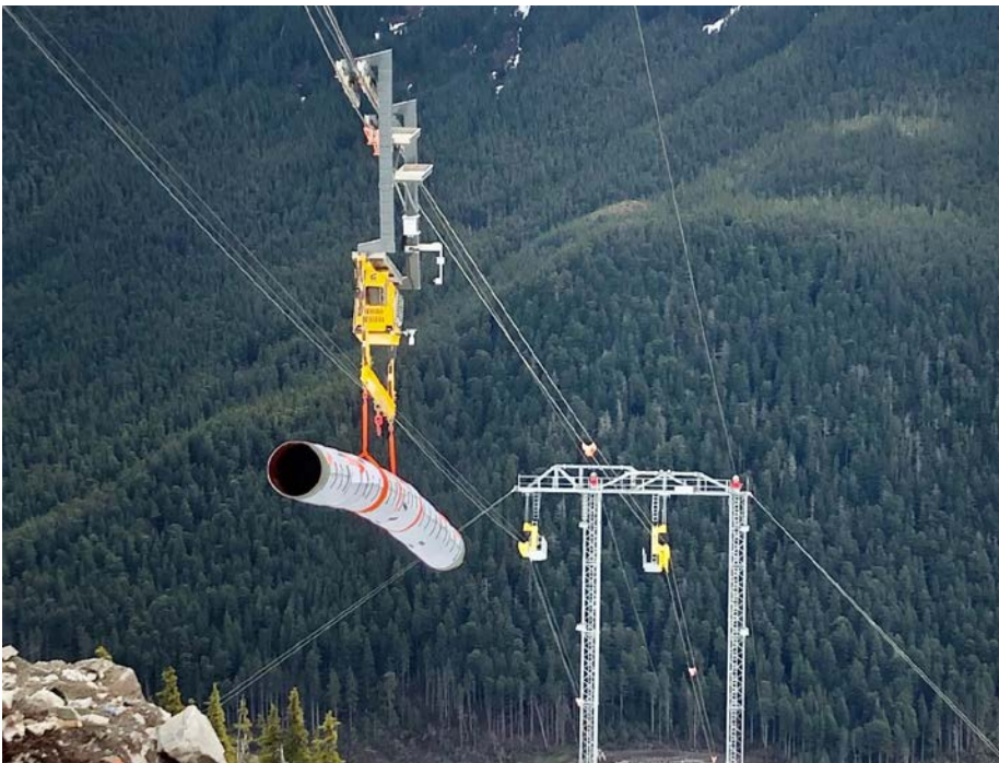
The epic cable crane in Section 8 West successfully traversed the steep slopes to deliver the first of an estimated 1,400 meters of pipe at Cable Crane Hill
