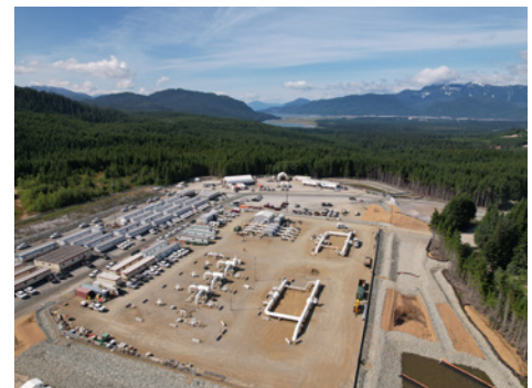
Aerial view of Kitimat Meter Station
