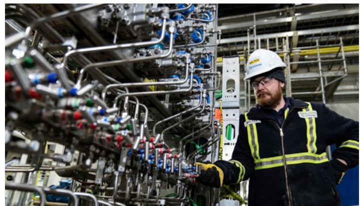
Employee adjusts manifold on Seal Gas Panel for compressor transmitters.
